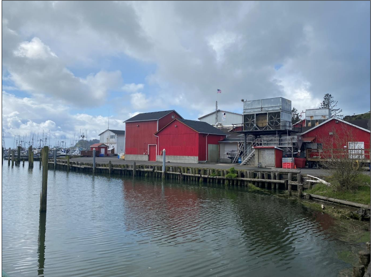
Figure 4. Overview of the East Bulkhead and Safe Coast Seafoods building with visible buckling of the bulkhead and asphalt. View is southwest.
