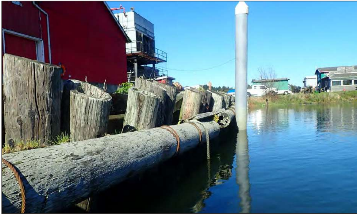
Figure 1. Damaged Bulkhead Wall
